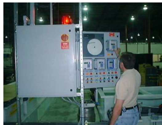
Water treatment system
